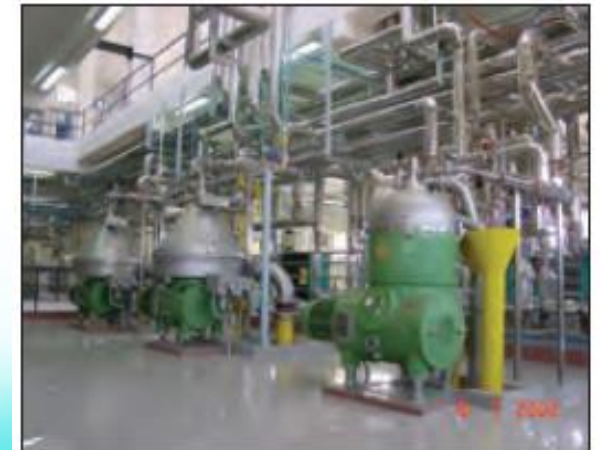
A piping network in an industrial facility.
