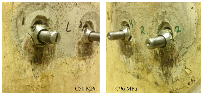
Fig. 25. Effect of plug concrete strength on slab spalling
